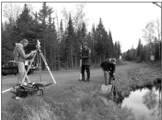
BRWA works with Paul Johnson (NRCS), Mike Pero (Ashland County), and Ted Koehler (USFWS) on culvert designs for Montreal Creek.
